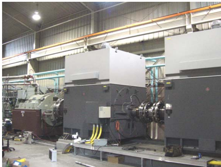
5 MW advanced prototype test facility for motors and converters
