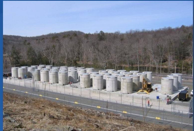
Dry cask storage for used fuel at the Surry station in Virginia
